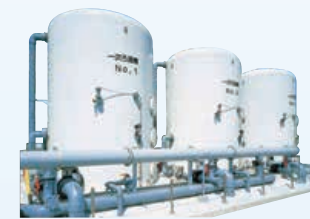
Sea Water Filtration Plants
