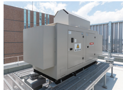
Standby generator used for the pilot operation
