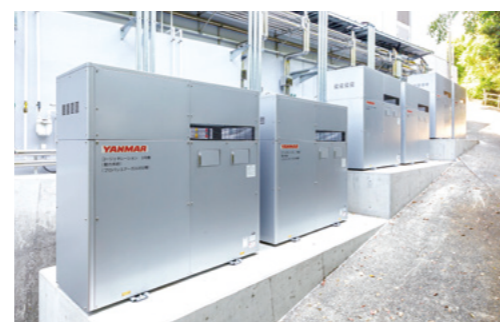
Cogeneration system installed at Hotel Ambia Shofukaku
