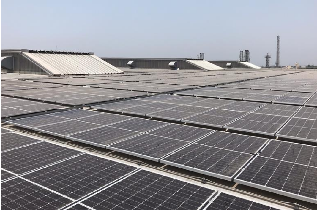
The solar panel installation at the Yanmar Engine Manufacturing India factory.
