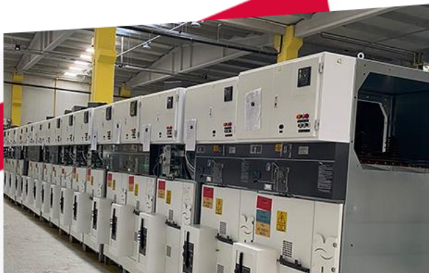
Steel Manufacturing, GUINEA
