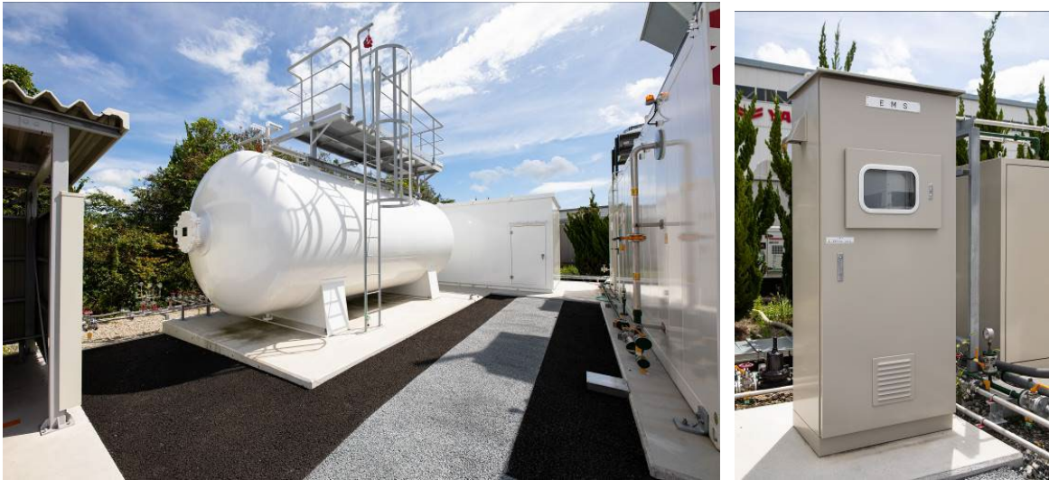
Left: Hydrogen Production Facility; Right: Energy Management System
