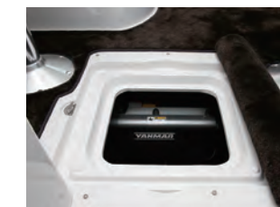
Cabin-side engine room hatch
